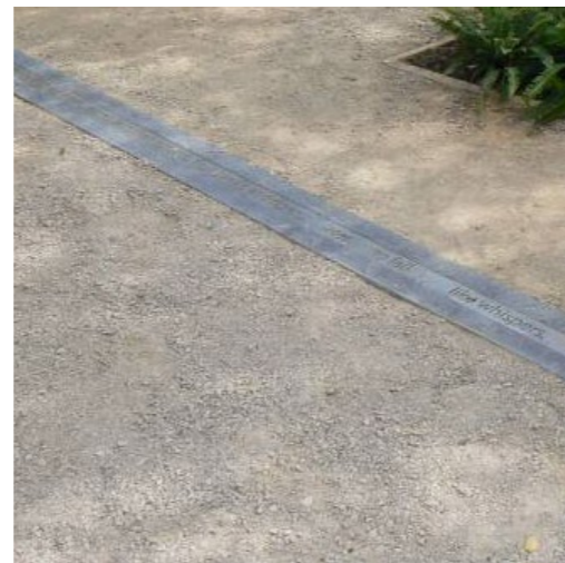
Pedestrian Paving 2 Market Square Self-binding gravel Size: 65mm depth compacted to 50mm depth Supplier: CED Ltd
