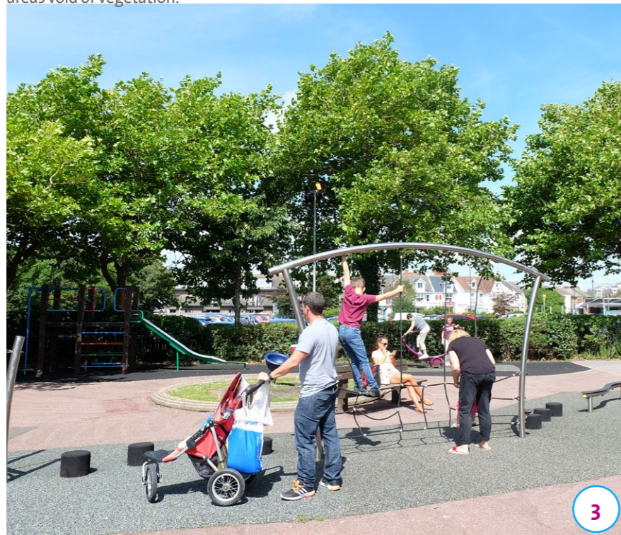
A well-used play area with relatively new equipment, however, the surrounding landscape and hard materials are poorly maintained with a patch-work of materials and areas void of vegetation.
